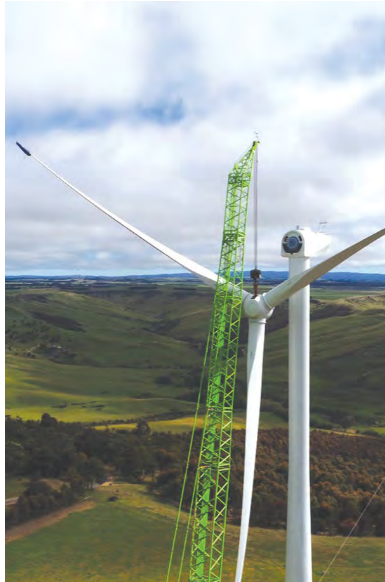
Right: A crane lifts a turbine rotor assembly into place at the Crowlands Wind Farm, two hours from Melbourne.
