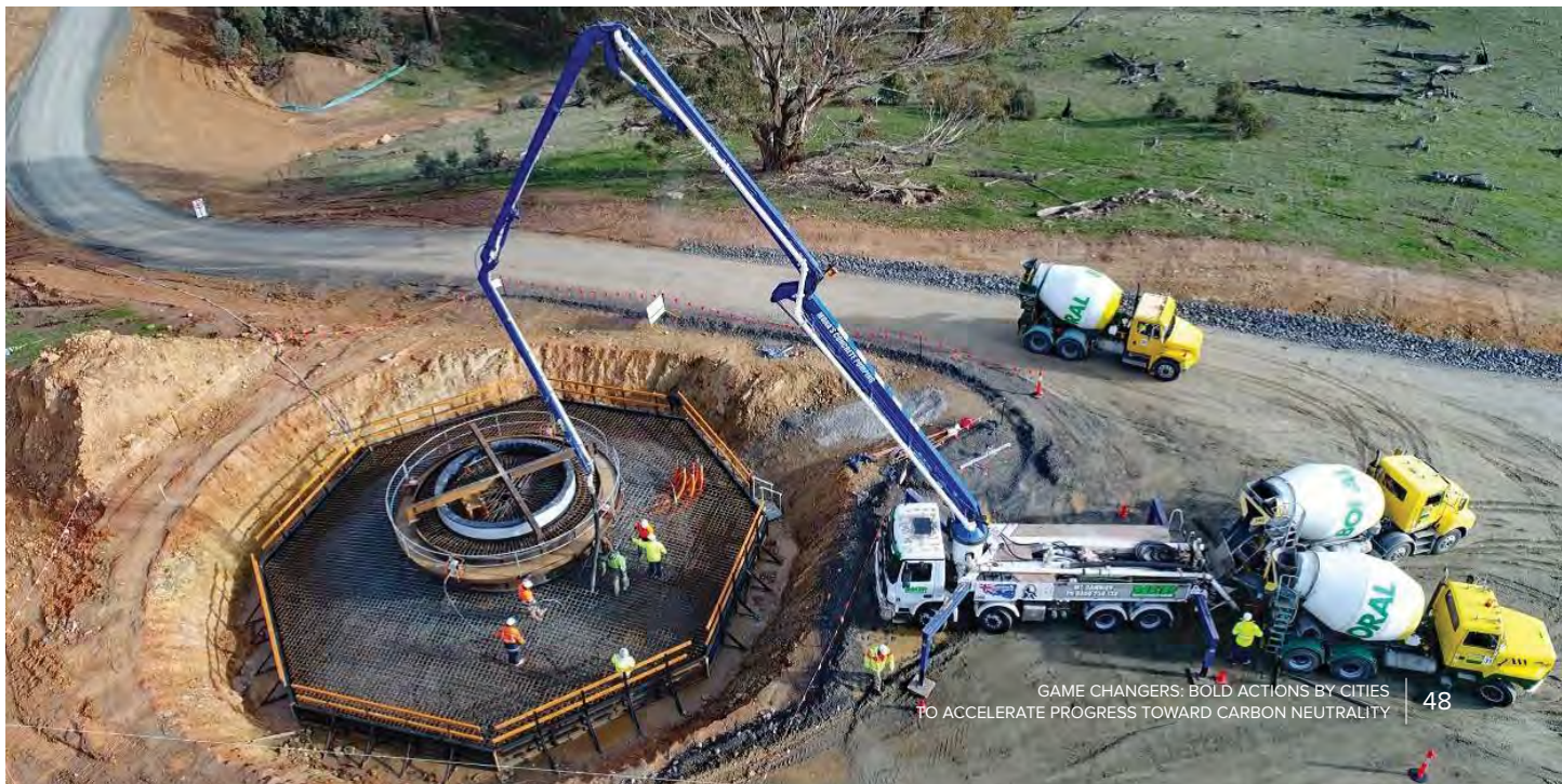
Below: Concrete is poured for the base of a wind turbine at the Crowlands Wind Farm.
