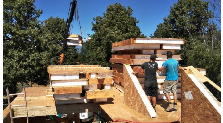
Lanefab Design/Build uses partially prefabricated framing using SIP panels for the framing of all of their projects.
