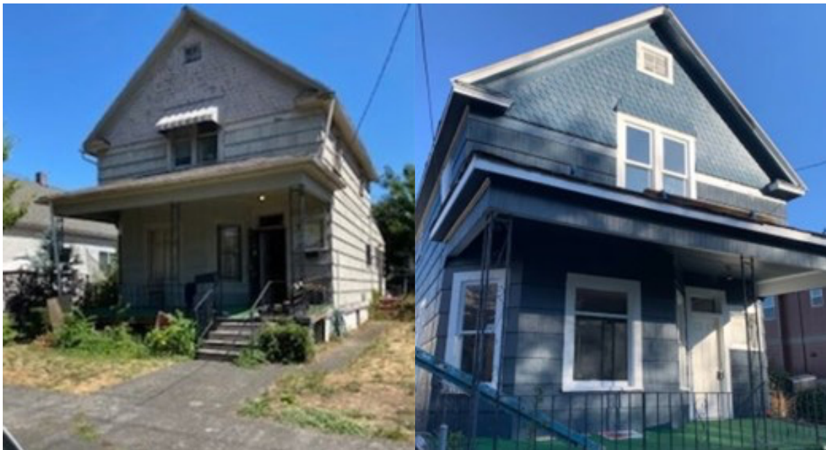
Image 4. BIPOC community members and those with disabilities receiving code violations in Portland, OR, can seek free assistance from the City. Pictured here is a before-and-after photo of a property. City of Portland
