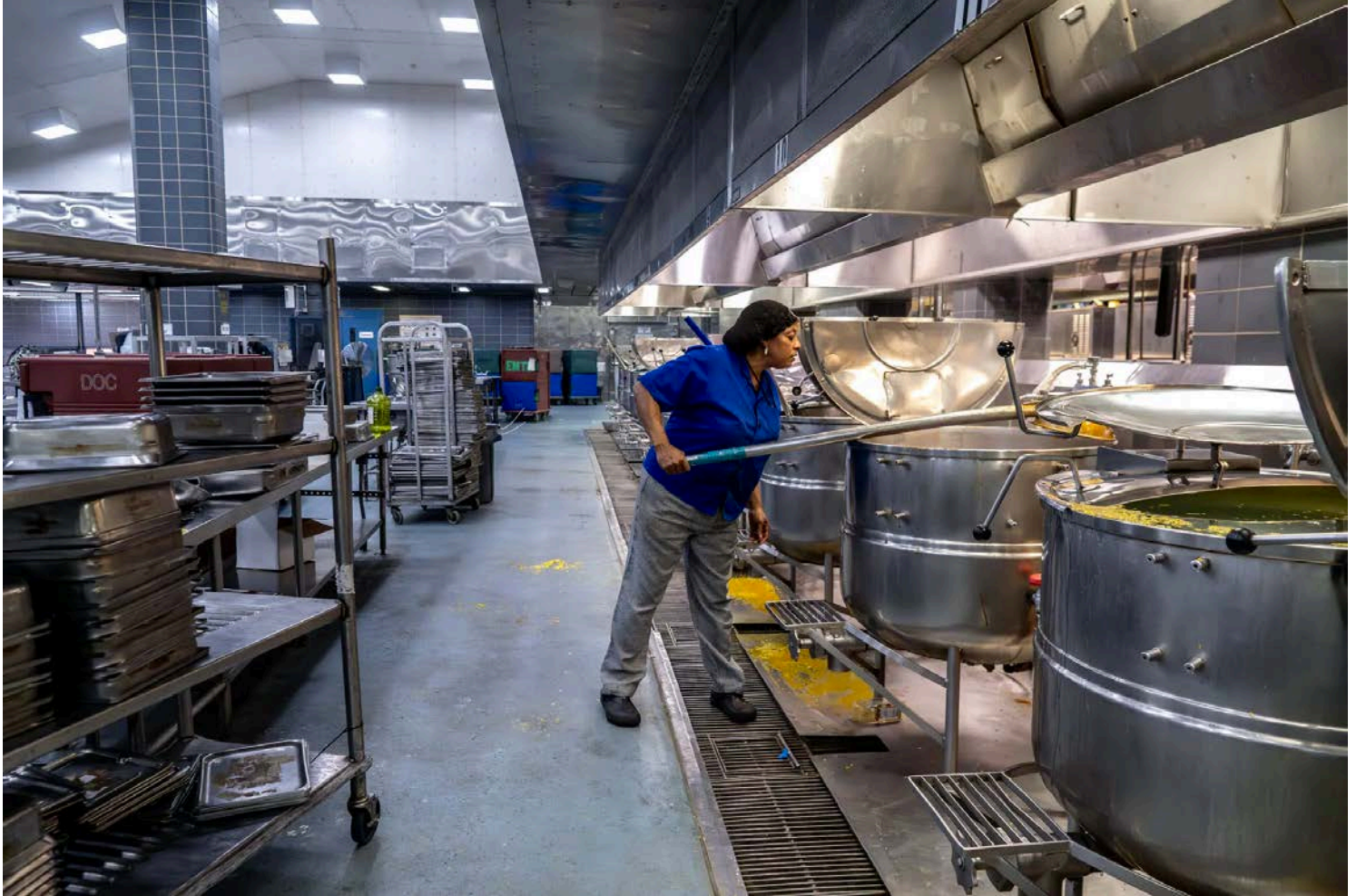
One of two kitchens on Rikers Island. It operates around the clock, and the cooks prepare every breakfast, lunch and dinner for detainees.
